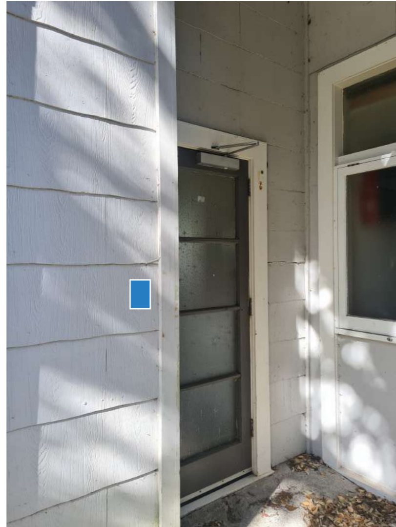
QR code by left side of door ACM Panel
