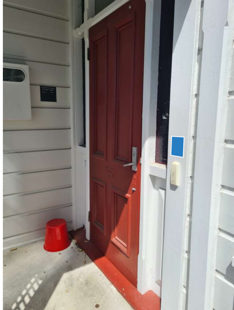
QR code by swipe access ACM Panel
