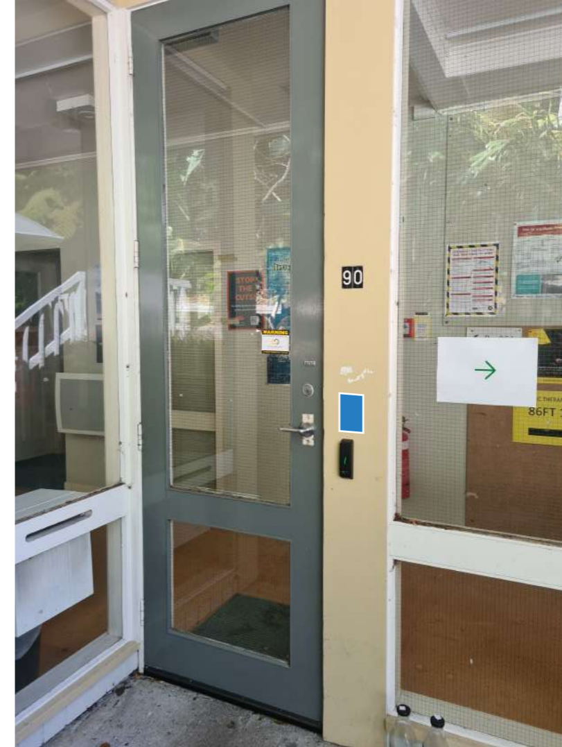
QR code by swipe access ACM Panel
