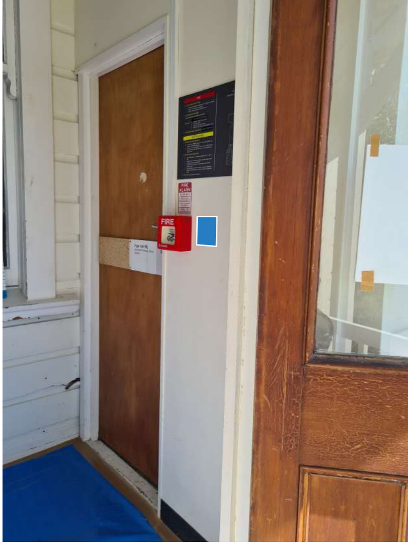
QR code by internal emergency signage ACM Panel
