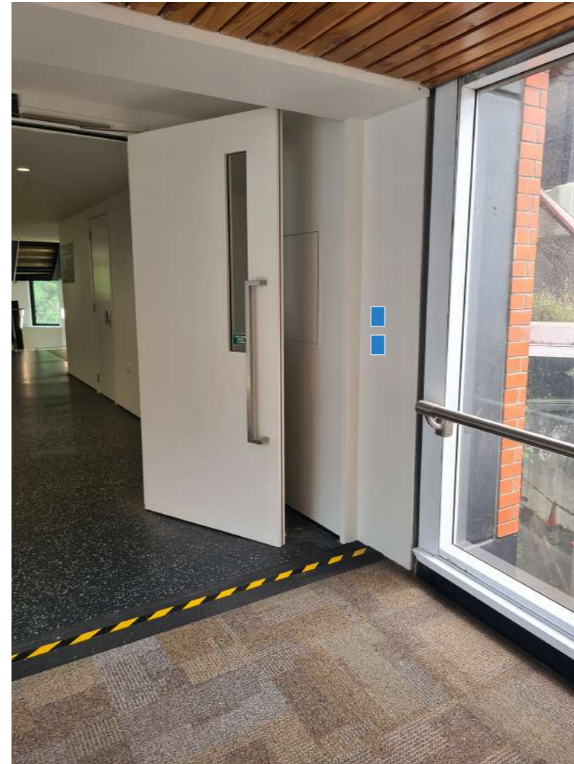
QR code by fire wall x2 - Bridge ACM Panel
