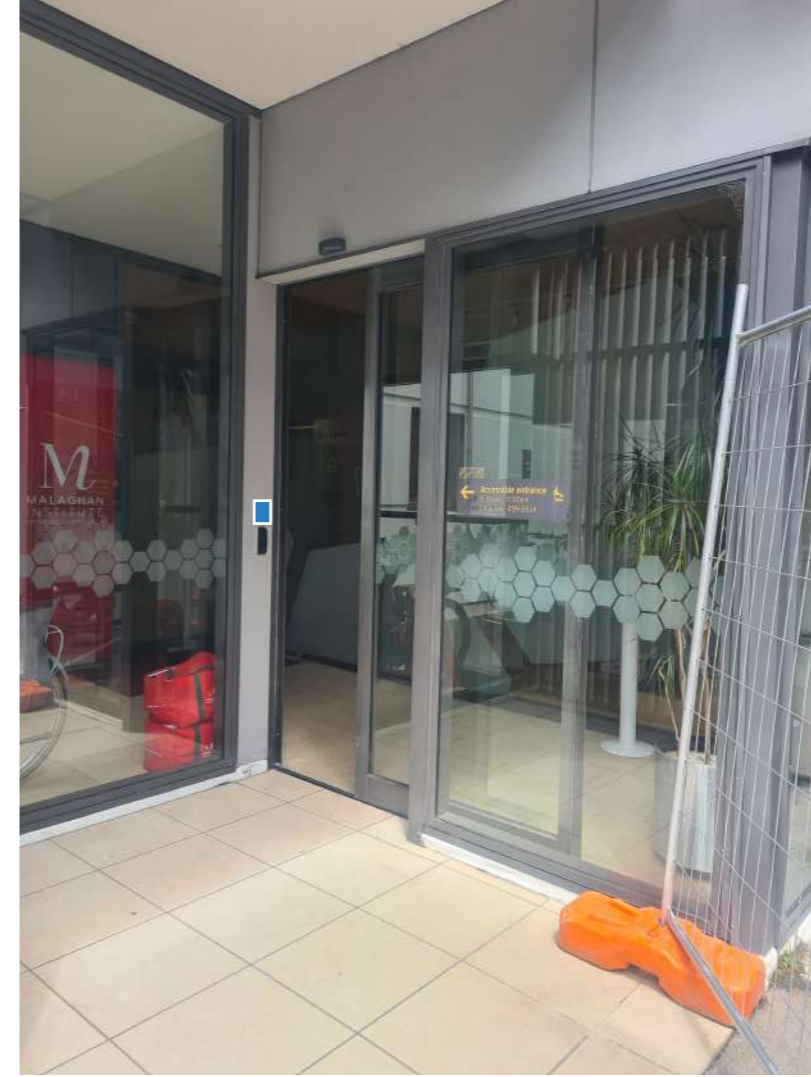
QR code by swipe access ACM Panel
