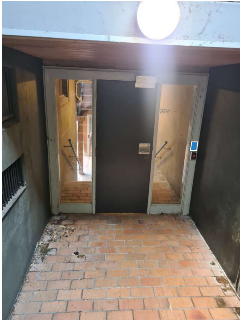
QR code by swipe access ACM Panel
