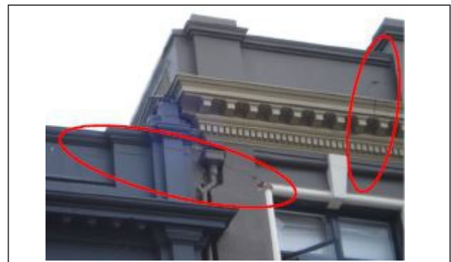
Fig. 9 Examples of URM pounding damage: minor damage.
