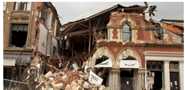
Fig. 16 Building collapse involving building pounding. Primary cause of collapse is attributed to URM construction. Photo courtesy of Colin Monteath, Hedgehog House.
