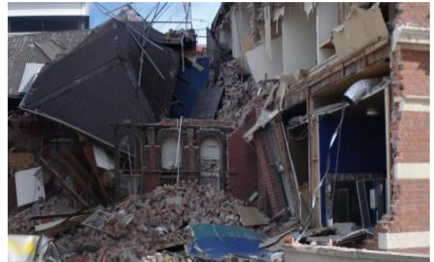
Fig. 15 Two storey building collapse involving pounding. Primary cause of collapse is attributed to URM construction.
