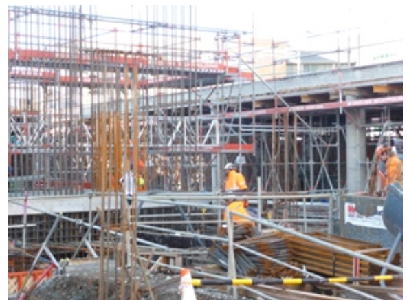
Fig. 2 Vertical reinforcement for the longitudinal structural walls can be seen on the left of the image.
