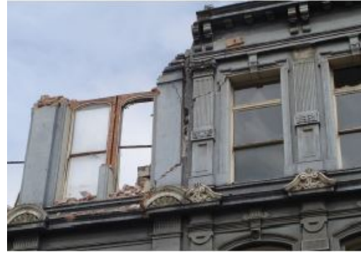
Fig. 10 URM: Major damage partially caused by pounding.
