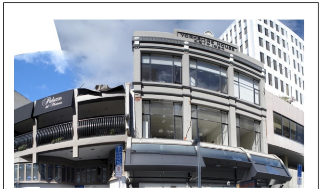
Fig. 14 Pounding damage caused by buildings with greatly differing heights. Note image is distorted due to panoramic photography.
