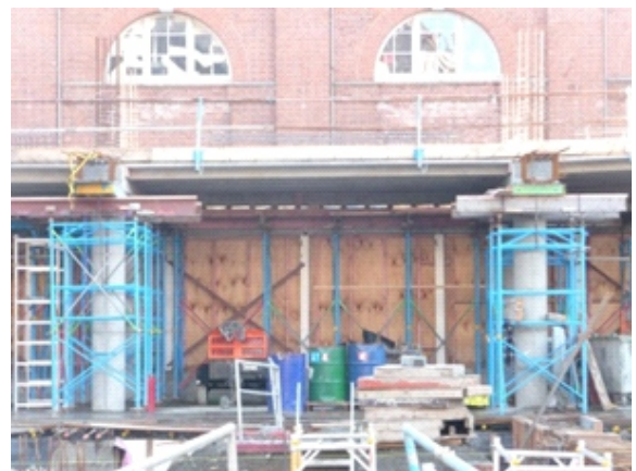
Fig. 3 A view of the gravity load-resisting columns and beams. Hollow-core slabs span between the beams.
