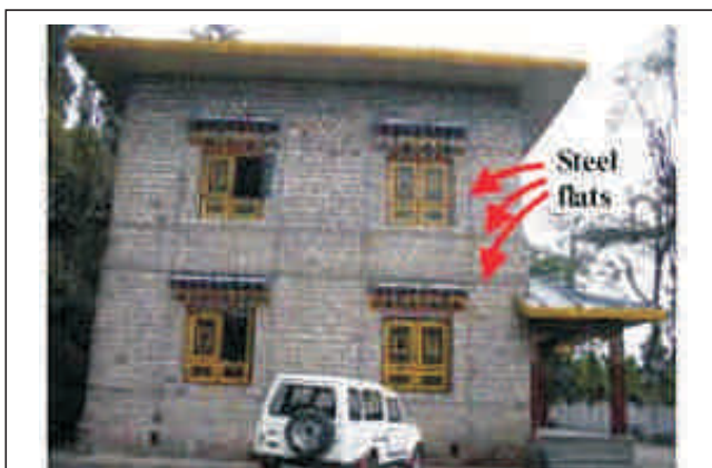
Fig. 5. Good performance shown by retrofitted Archive building (arrows show steel flats used to retrofit the building after the 1988 Bihar–Nepal earthquake).
