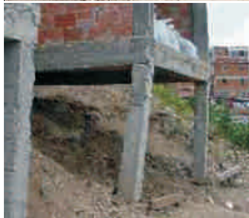
Fig. 11. Flexural failure of short column (above) and flexural failure of long column (below) of Model 1.
