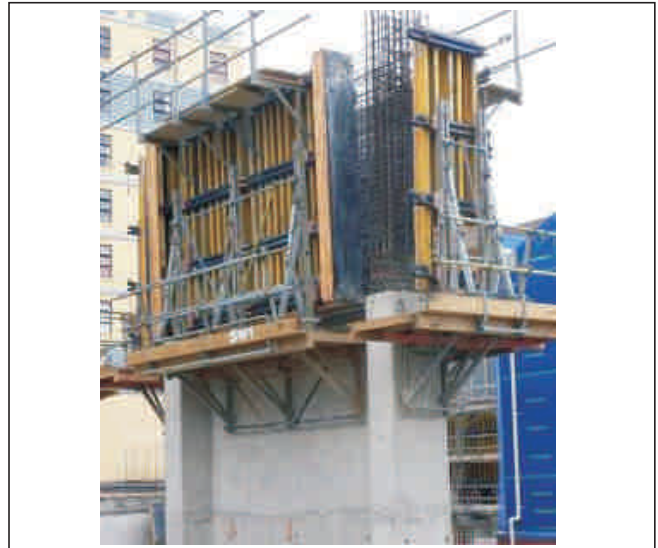
Fig. 2 A wall with its formwork open to reveal the reinforcing layout at the end of the wall.
