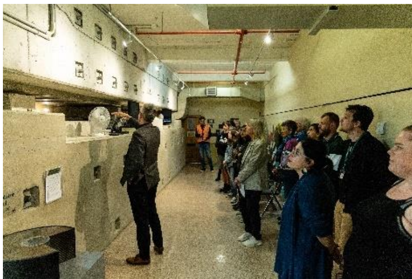
Engineering expert Hamish McKenzie explains the workings of Parliament's base isolators.
